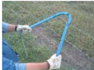
Step 1. Choose any convenient point along the slack fence line to make the repair.
